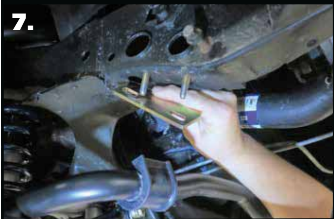
7. Install a 5/16" flat washer on each of (2) 5/16"-18 x 1 1/4" bolts and insert them into the OEM sway bar holes by inserting them in through the access holes in the side of the frame. Install the spacer plate with the wide side positioned to the inside. Hold it in place.
